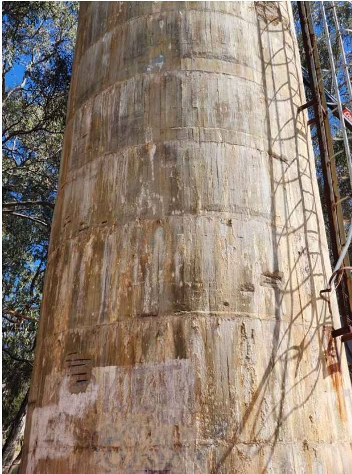
Example of leachates at horizontal construction joints (concrete pour stops)
