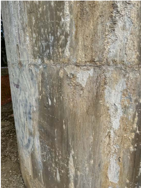
Example of efflorescence/calcium salt deposits on surface of concrete
