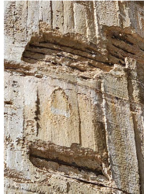
Examples of concrete section loss and severe reinforcement corrosion and section loss on external wall
