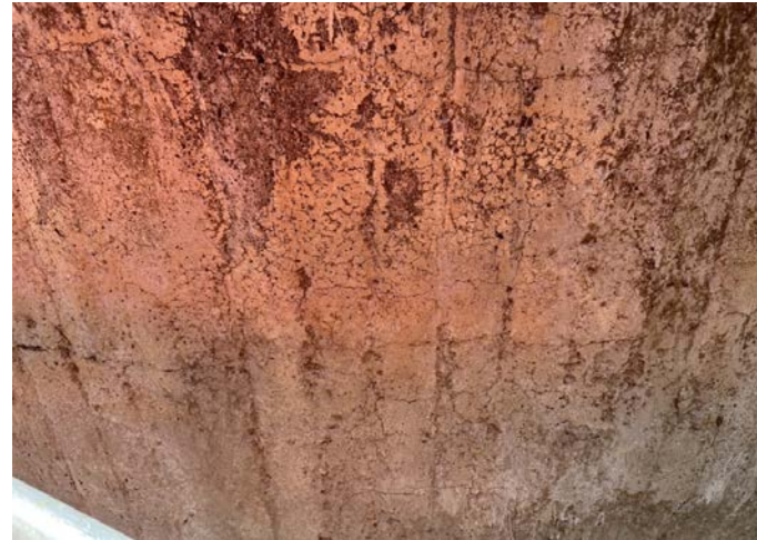
Examples of cracking which was characteristic of structure
