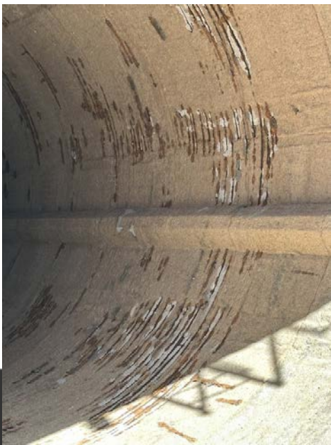
Internal wall example of widespread reinforcement corrosion
