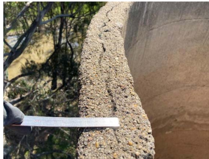
Examples of cracking present at top of tower
